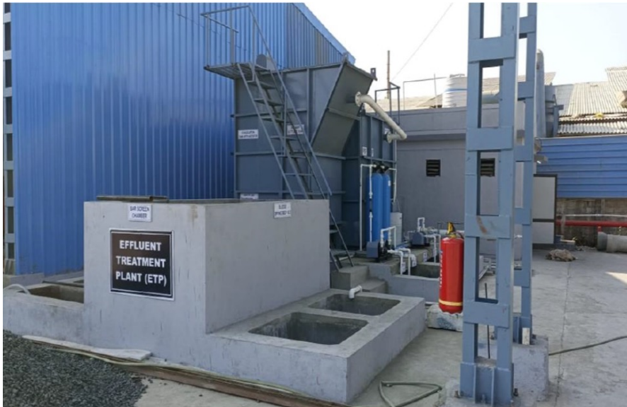
15 KLD ETP Plant at Gandhidham - Kachchh, Gujarat
