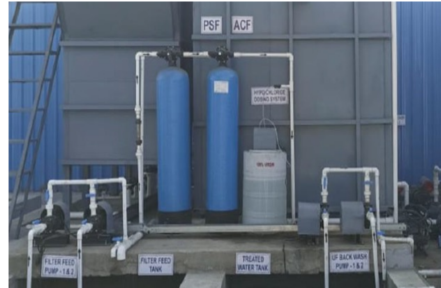
Pressure Sand Filter and Activated Carbon Filter systems
